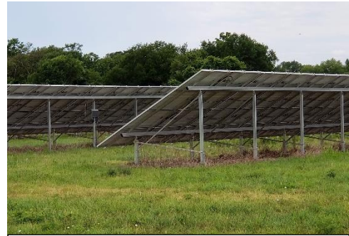
Example of a Solar Conversion System, Ground-mounted
